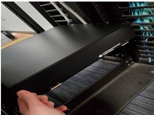
Figure 13: Cover Replaced on front of panel
