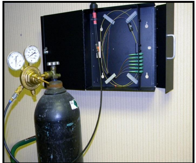
Figure 8 Ready Gas Bottle at Entry Point FTU
