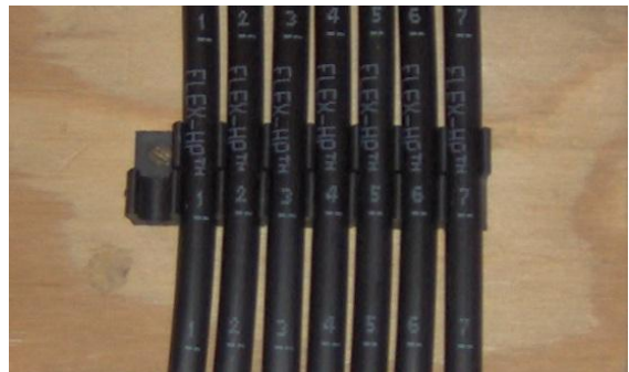
Figure 9b Tubes Neatly Organized and Secure
