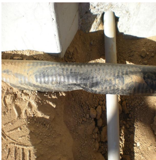
Figure 1 Damaged Tube Cable
