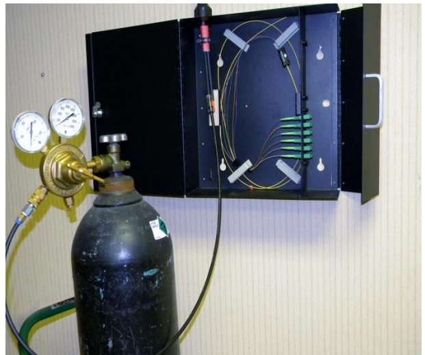
Figure 8 Ready Gas Bottle at Entry Point FTU
