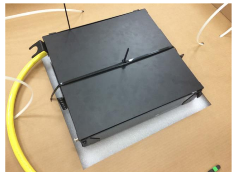
Figure 11 Tie Down Securing Patch Panel
