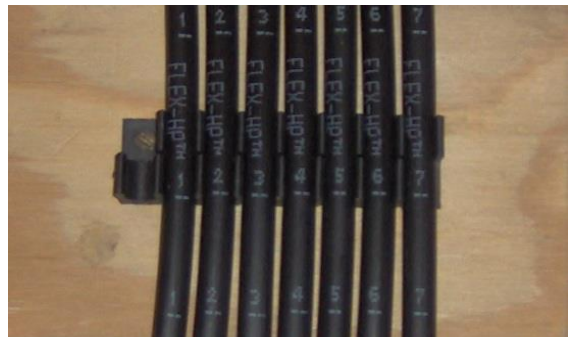
Figure 9b Tubes Neatly Organized and Secure
