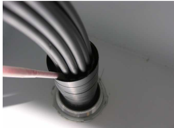
Figure 20a Injecting Epoxy Sealant in Open Space Between Outer Ring Tubes and Encapsulant Container
