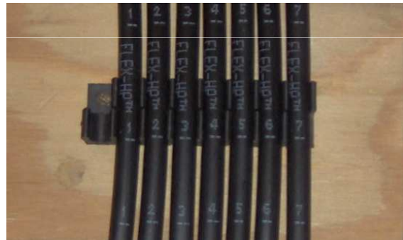
Figure 9b Tubes Neatly Organized and Secure
