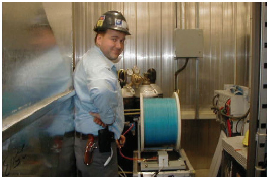
Blown fiber requires only two installers—one at each end of a splice-free continuous fiber run. This modest personnel requirement eliminates large work crews and disruption.
